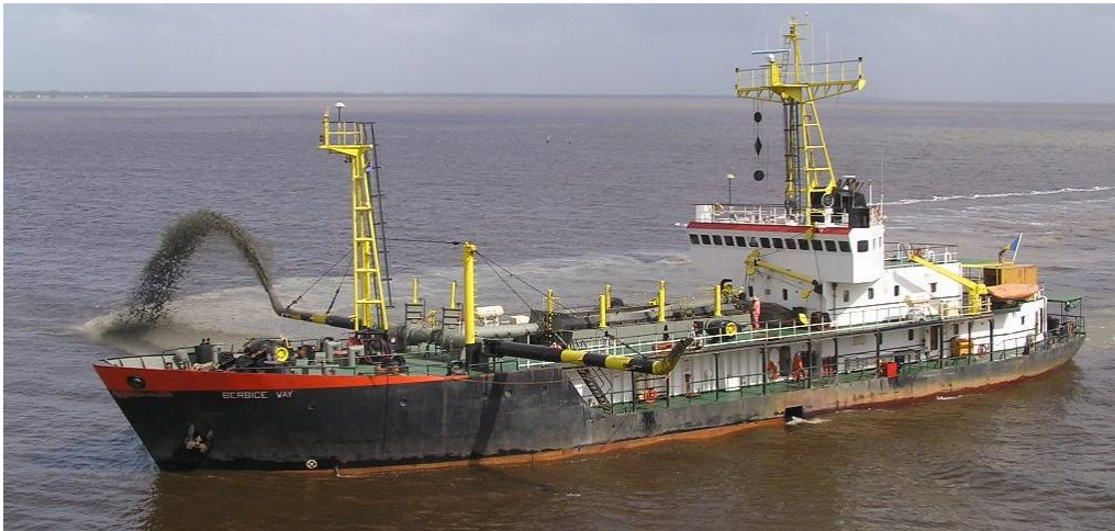
Dredging the Fairway on the Berbice River to New Amsterdam (Guyana) April 2008 © Captain Peter / Shipspotting
