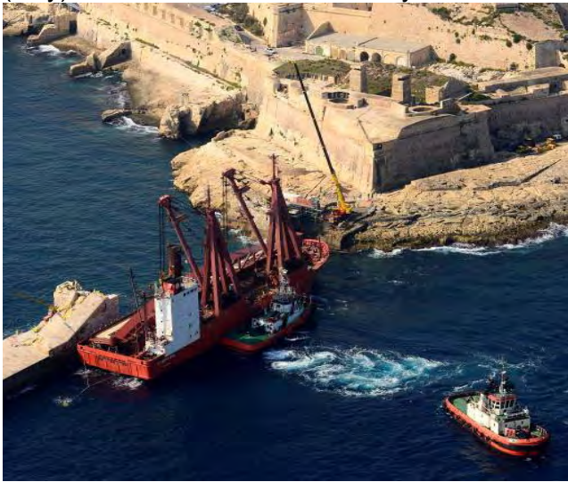
The Storman Asia is erecting the bridge over the local breakwater in Valletta (Malta), October 2011 © Airphotomalta / Marinetrffic
